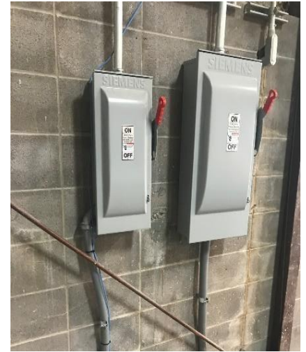
Figure 1: 480VAC Electric Disconnects
