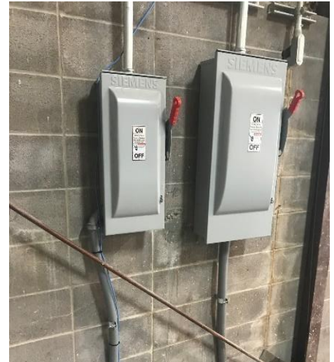
Figure 1: 480VAC Electrical Disconnects
