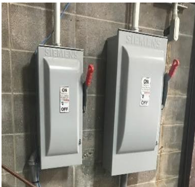
Figure 1: 480VAC Electric Disconnects
