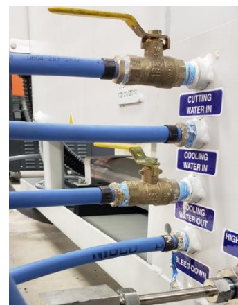
Figure 5: Waterjet Pump Plumbed (Example)
